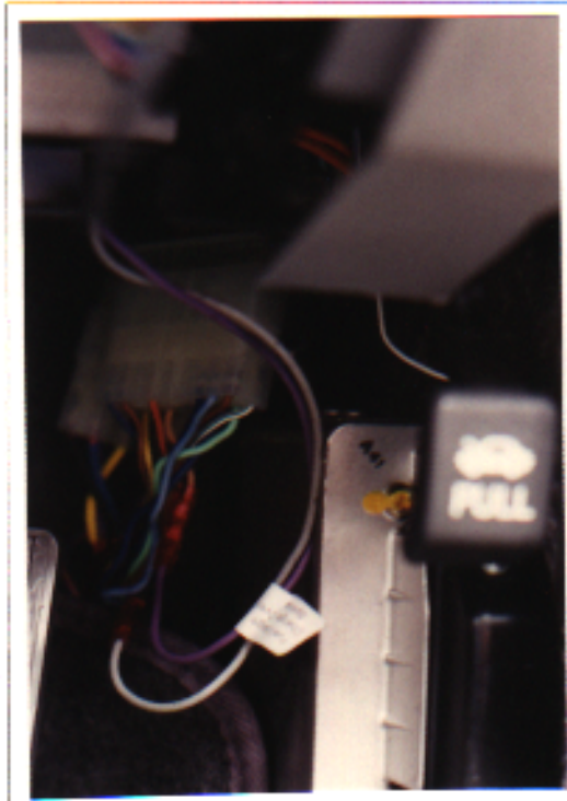
Fig. 19 RHS Door Pillar Showing Fuel Gauge Splice and LPG Fuse.
